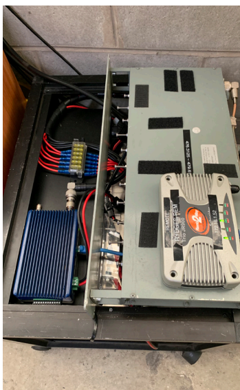
Each cnReach N500 radio linked NXDN trunked repeater sites. Renta 2-Way added a fully featured IP console which operated at full capacity.
